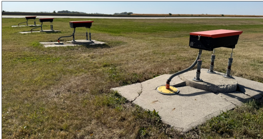
A set of PAPIs that will be replaced with the project
